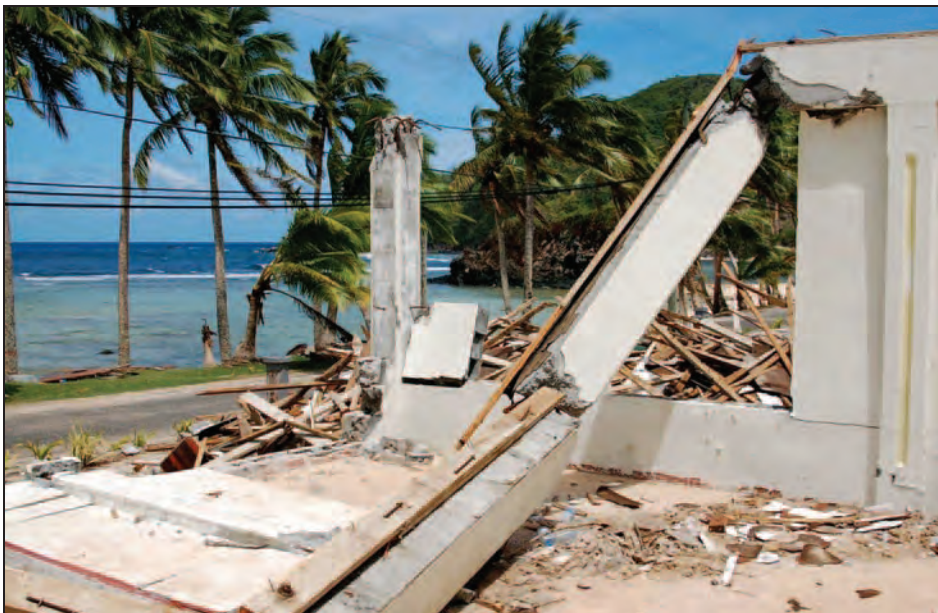
Figure 3-12. Damage from the 2009 tsunami (Amanave, American Samoa)
