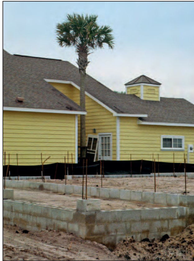
Figure 4-25. (below) Notching the building and roofline around a tree can lead to roof and envelope damage during a high-wind event
