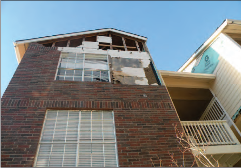
Figure 3-11. Apartment building with gable end wind damage from Hurricane Ike as a result of poor connection between brick veneer and wall structure (Galveston, TX, 2008)
