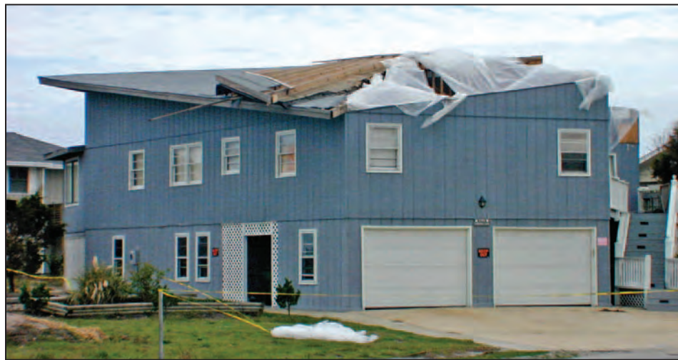
Figure 4-4. Although sited away from the shore, winds from Hurricane Floyd (1999) tore off the large overhanging roof of this house in Wrightsville Beach, NC
