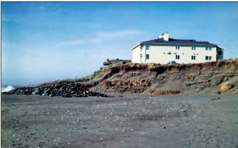
Figure 3-42. Buildings threatened by erosion at Ocean Shores, WA, in 1998. The rock revetments were built in response to shore erosion along an area adjacent to a jetty and thought to be accretional
