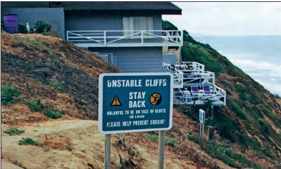
Figure 3-51. Unstable coastal bluff at Beacon's Beach, San Diego, CA
