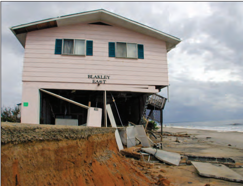
Figure 3-33. Erosion undermining a coastal residence in Oak Island, NC, caused by Hurricane Floyd in 1999
