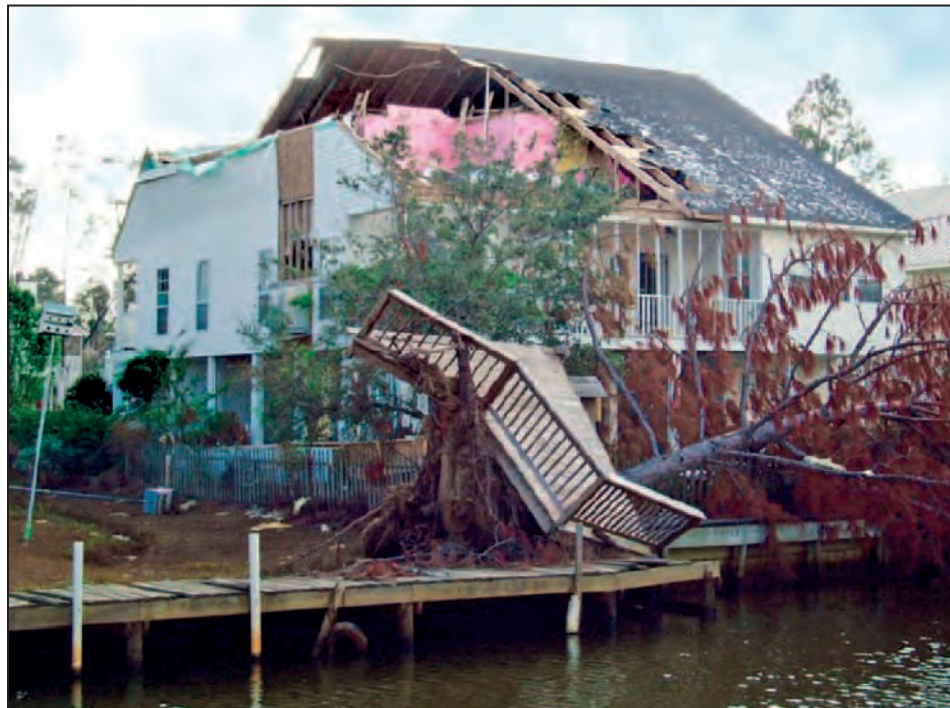
Figure 2-17. Wind damage to roof structure and gable end wall, Hurricane Katrina (Pass Christian, MS, 2005)
