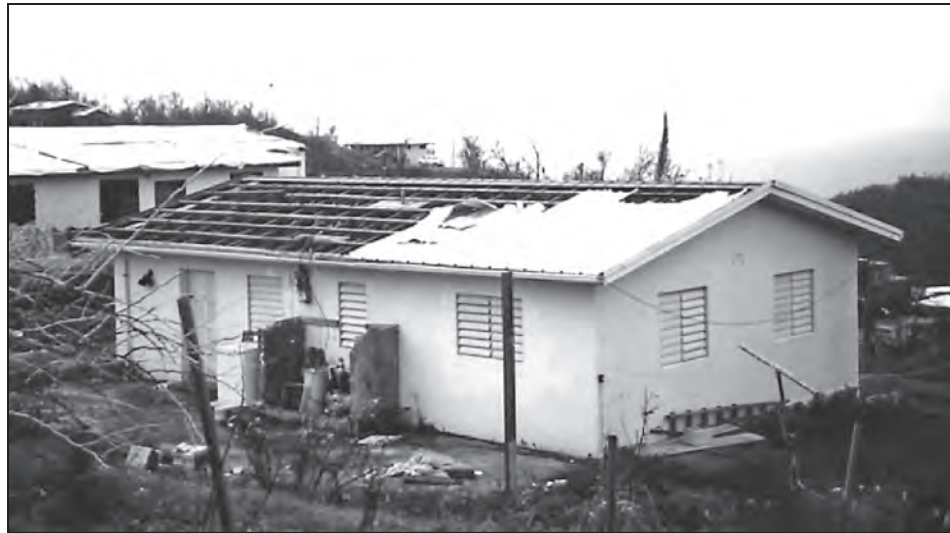
Figure 2-6. This house lost most of its metal roof covering due to high winds during Hurricane Marilyn in 1995 (location unknown) SOURCE: NRCA 1996
