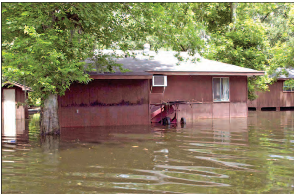
Figure 3-4. Storm surge flooded this home in Ascension Parish, LA (Tropical Storm Allison, 2001)
